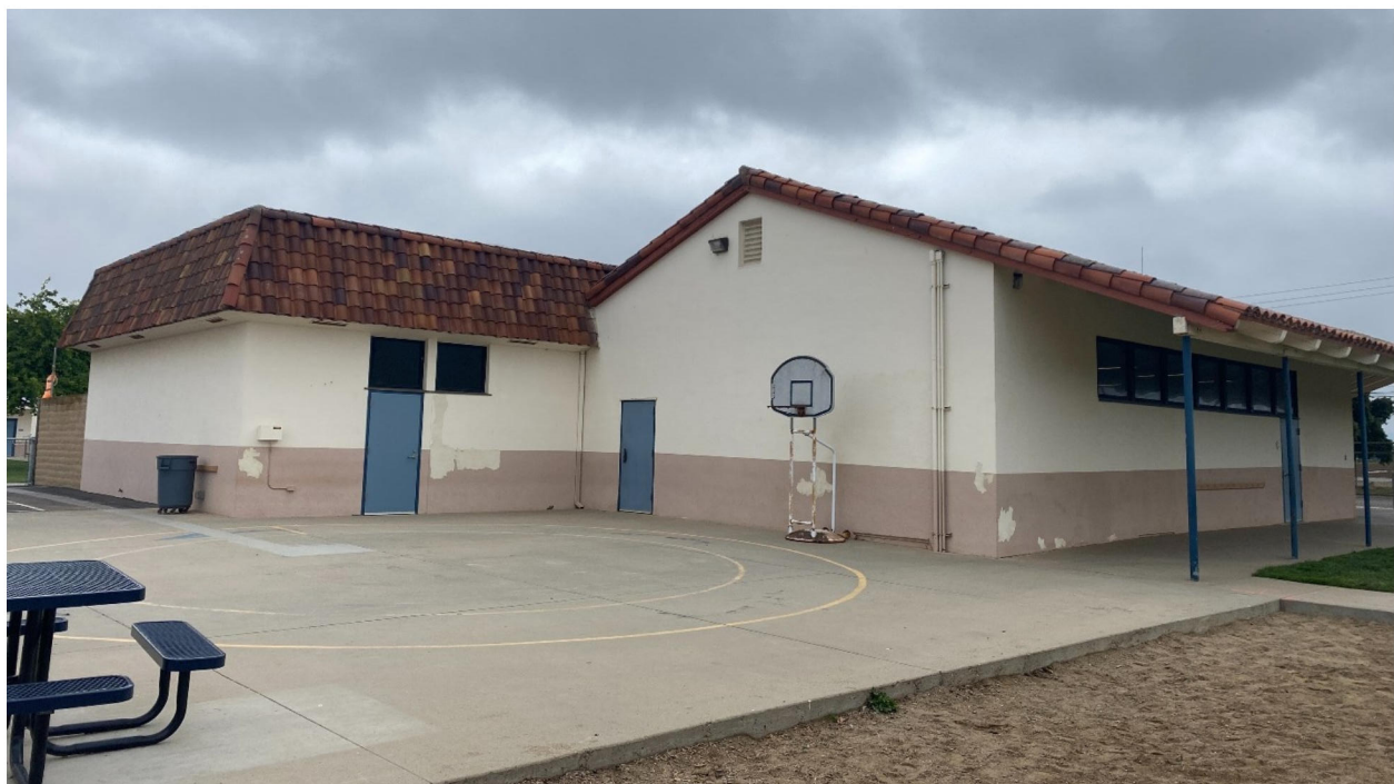
Photograph 8. South and west elevations of Bonita Elementary School Kindergarten Building, view northeast.
