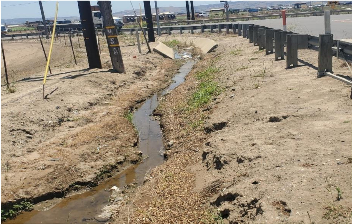
Photograph 1. Photograph of the ditches on the east side of Bonita School Road, facing south. June 28, 2023.
